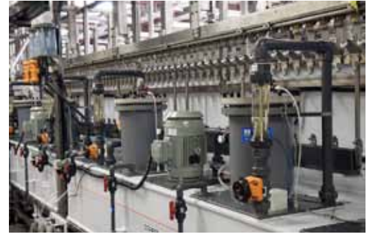
Easy access utilities and service area
